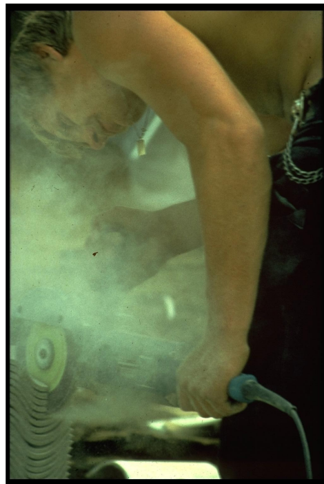
Figure 3. Example of a working posture linked to the high asbestos dust levels typical of this job, illustrated here by a young roofer cutting off the edges of corrugated asbestos cement roof slabs using a disc cutter at a construction site in 1978. Approximately 60 million chrysotile asbestos fibers per cubic meter of air were measured in this workplace (see also another example of health impact of such exposures on a case report in chapter 3 of the Appendix).
